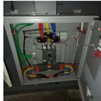
(AC Side Termination)
