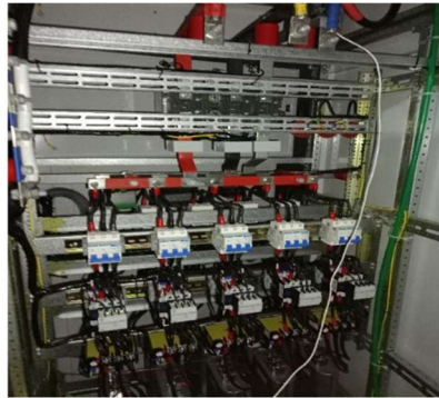
(Capacitor Bank Termination)
